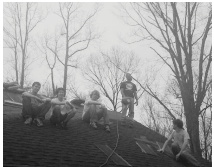
Brothers Clarke, Tao, Paulzak, Tharakan, and Culbert repairing a roof at the local Boy Scout camp in Spring 2009.
